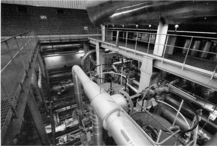
One of the two newer generator halls (3 or 4). They have been converted to run on light diesel fuel and are still in the Swedish national reserve to start up in cold climate. Burner and boiler to the right and the generators to the left
